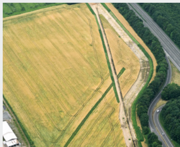
Figure 4: A double HDD pipe string (black polyamide coat) with a test pipe specimen welded to its front end is ready for pulling through the bore. The conventional double pipe string (yellow coating) is ready for lowering into the trench
