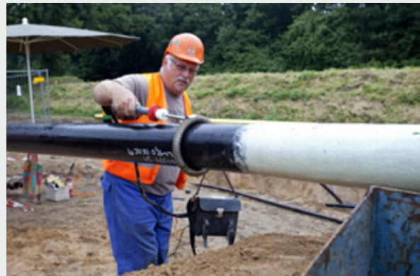
Figure 2: Before pulling in a pipe string, the pipeline constructors always subject the coating's quality to a special test
