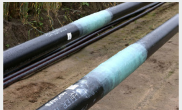
Figure 8: In the Zephir project, a combined PE-GFRP system is used for field coating
