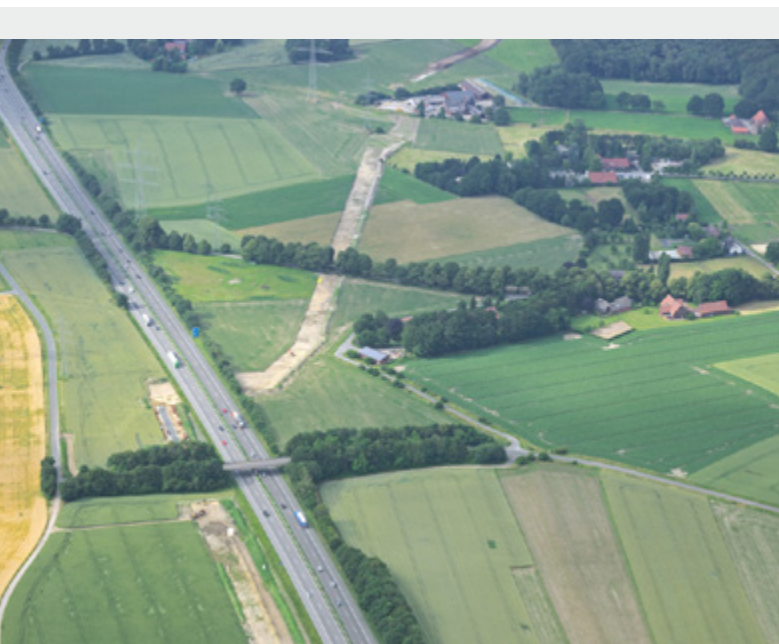
Figure 1: For the underground crossing of the A 52 freeway, Köster GmbH used a pipe jacking technique in which a DN 800 steel-in-steel pipe to protect the product pipes inside it was hydraulically pushed through the soil
