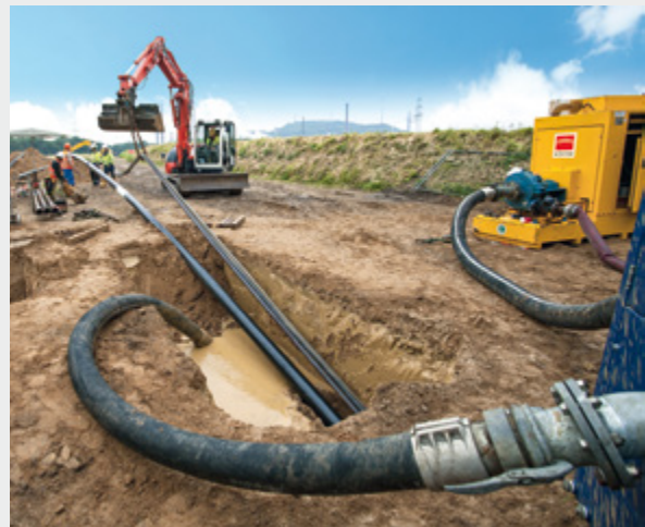
Figure 3: To support HDD bores, a liquid clay mineral mix – bentonite – is used
