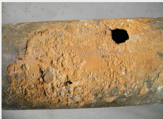
Figure 7: Corrosion damage in a first-generation ductile iron pipe
