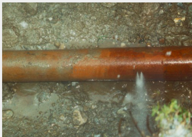
Figure 6: Corrosion damage in steel pipe
