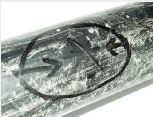
Figure 3: Crack in an embrittled PE pipe on a point support
