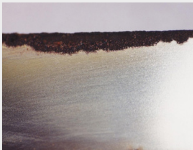
Figure 4: Graphite corrosion in a gray cast iron pipe
